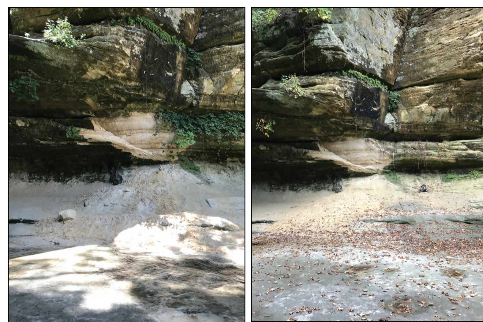
In 2017 and 2018, rockfalls occurred demonstrating the natural potential for changes to bedrock surfaces an hazards in this environment. Visitor traffic to the area aided in transportation of loose sediments and breakdown of larger fallen blocks. Monitoring all surface changes helps communicate hazards, safety, and preservation.
